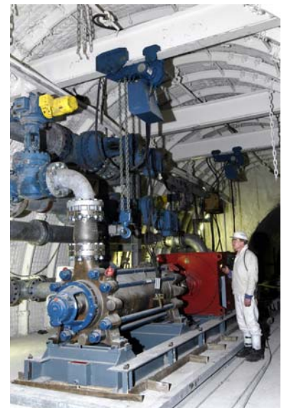
Maintenance work in a pump station. In operation: 8 JDN Air Hoists Profi 6 TI in motorised Low Headroom Trolleys.
